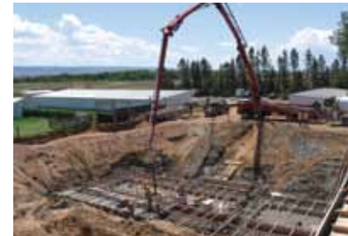
New veterinary laboratory addition on the campus of the University of Wyoming in Laramie, Wyoming.
