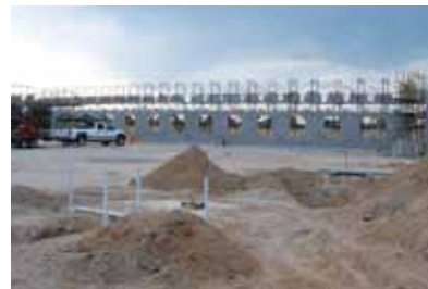
New public health lab, environmental quality lab and criminal investigation lab is underway in Cheyenne, Wyoming.
